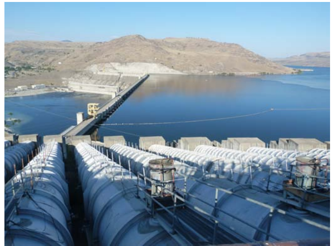
The John W. Keys III Pump Generating Plant would be upgraded under new provisions. Photo: K.C. Mehaffey
